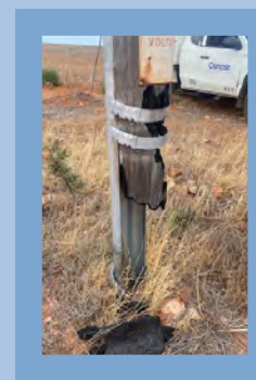
Catastrophic fire damage to trussed pole
