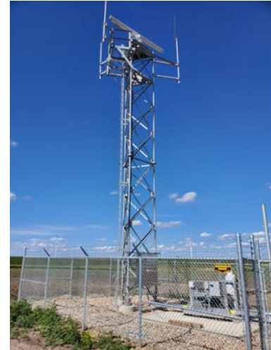
Figure 2: Typical ADLS radar and tower installation
