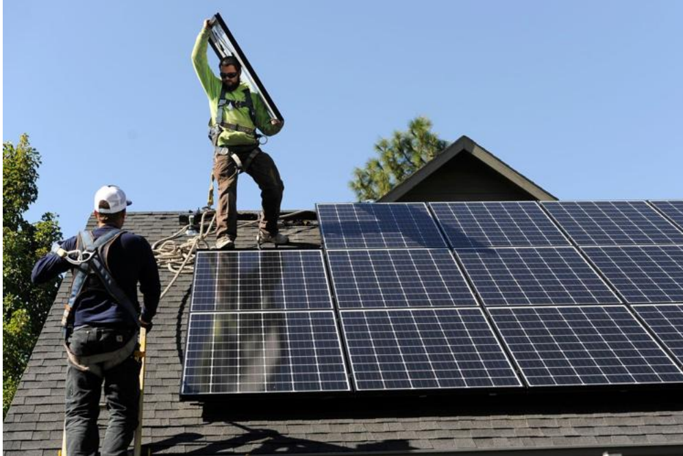
Workers install a solar system for a Bend customer on Wednesday, Oct. 4, 2017. (Ryan Brennecke/Bulletin file photo)
