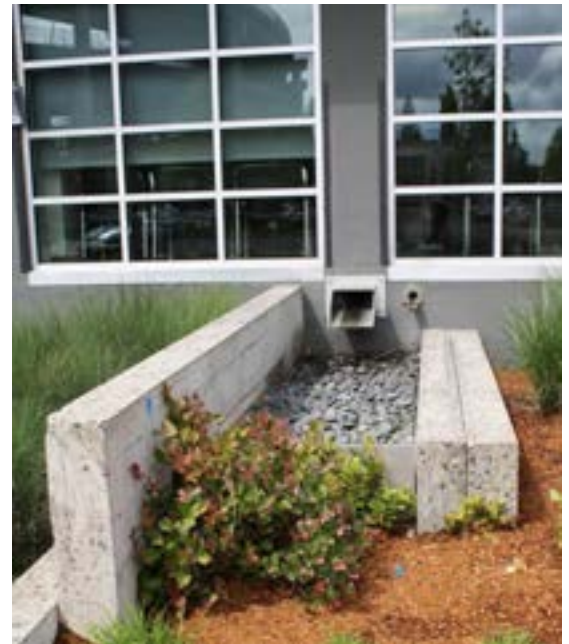
Disconnected Downspout, Rivereast Center, Portland, Oregon, by.
