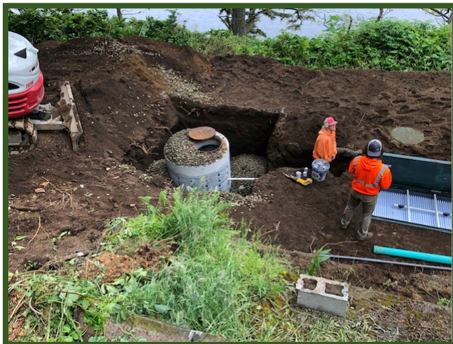
Left: An approved alternate treatment (ATT) septic system is installed near a waterway in Tillamook County. - Photo provided by Tillamook County
