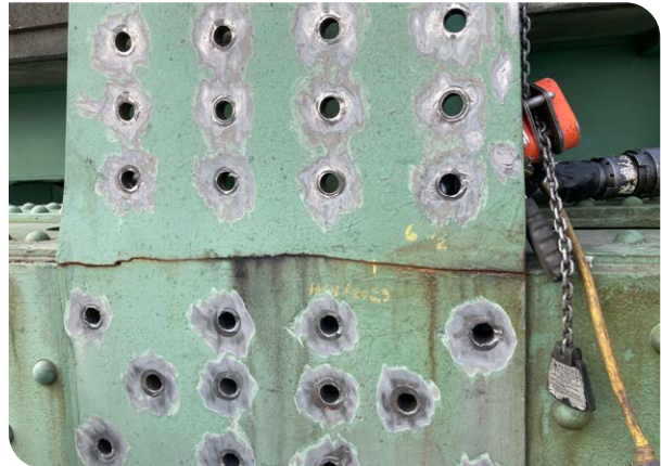
Steel Fatigue Crack
