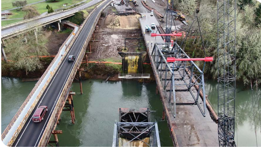
Van Buren Bridge – Removing the old bridge while traffic was shifted onto the diversion structure.
