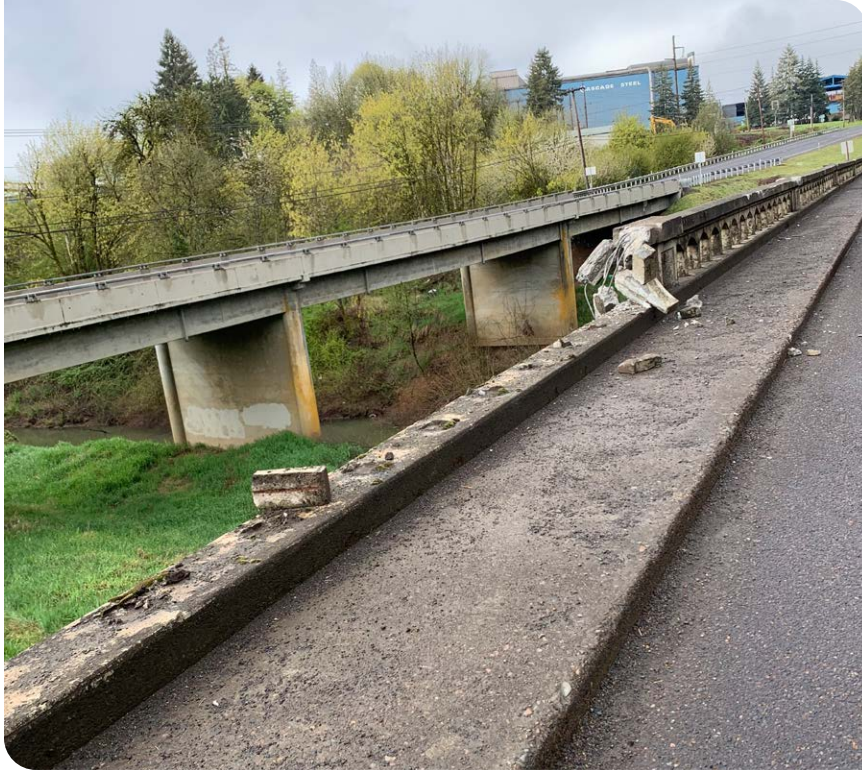
In April 2024, a vehicle lost control and impacted the bridge rail. A significant portion of the bridge rail was demolished. Fortunately, the vehicle was able to remain on the bridge.
