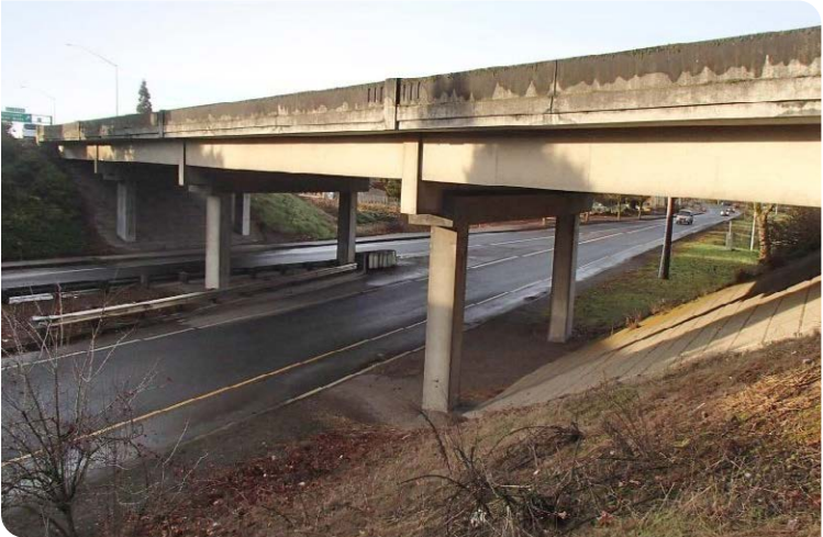
This Interstate Era Bridge is one of four bridges at the North Albany Interchange where I-5 crosses over Oregon 99E.
