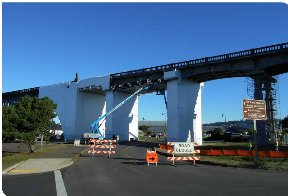
Temporary work access and containment on the Yaquina Bay Bridge (Newport, OR) – Cathodic Protection Work (2023).
