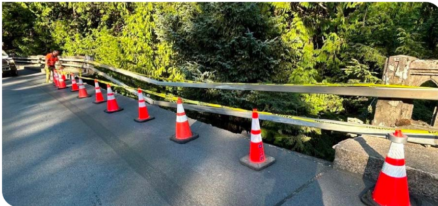
Necarney Creek Bridge on U.S. 101 shows a significant portion of the sidewalk and bridge rail has failed. The two rectangular tubes that were added in 2008 are the only barrier that remained after the vehicle impact.
