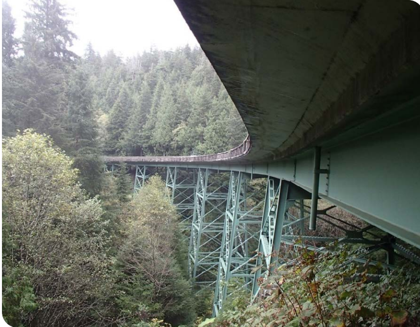
The Necarney Creek Bridge has a significant curve and Necarney Creek is in a deep valley.
