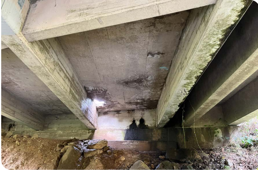
The I-5 northbound bridge over Elk Creek is located south of Cottage Grove.
