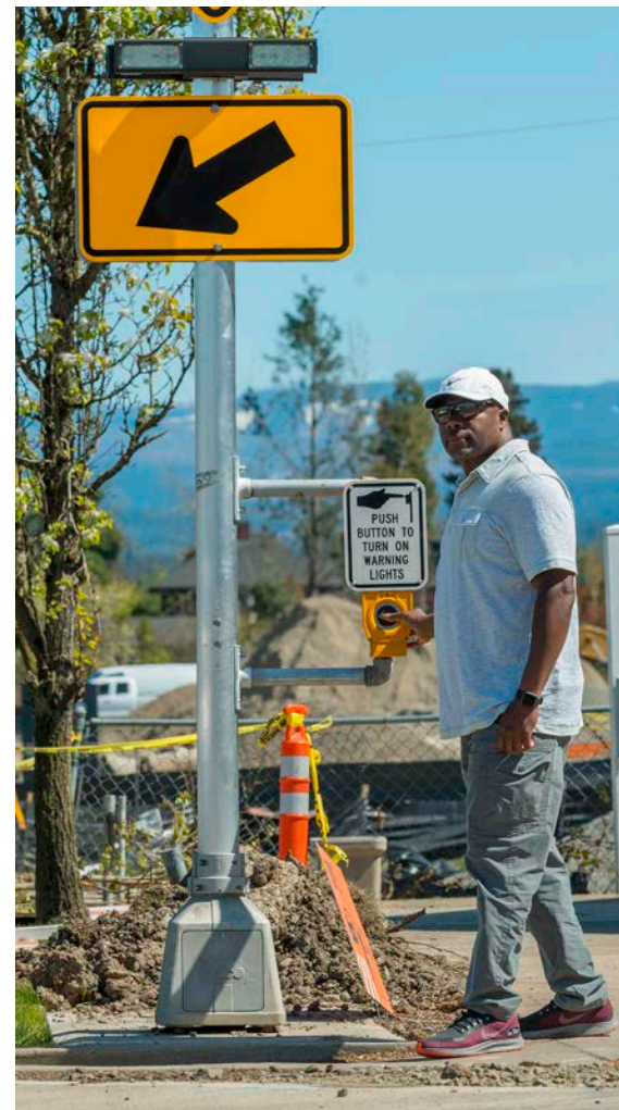
A minimum of $9 million per year is needed to address deficiencies at marked crosswalks.
