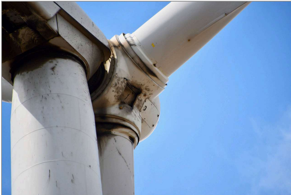
A Vestas V82 turbine, missing a hatch door, at PGE's Biglow Canyon wind farm this summer. Farmers say the hatches fall into their fields from a height of 265 feet. (Courtesy Kathryn McCullough)
