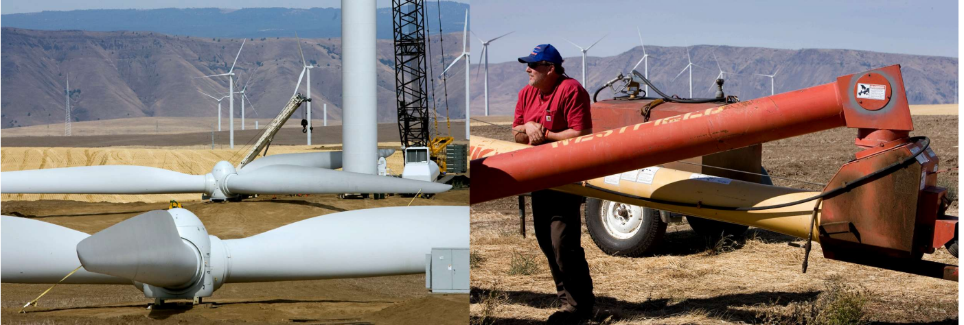
The first 76 Vestas turbines under construction at Biglow Canyon wind farm in 2007. Kevin McCullough, right, looked on enthusiastically at the time. He farms under about half of the wind farm's 217 turbines today and earns lease payments based on electricity production from the 13 turbines on land he and his wife own there. (File photos by Ross William Hamilton)
