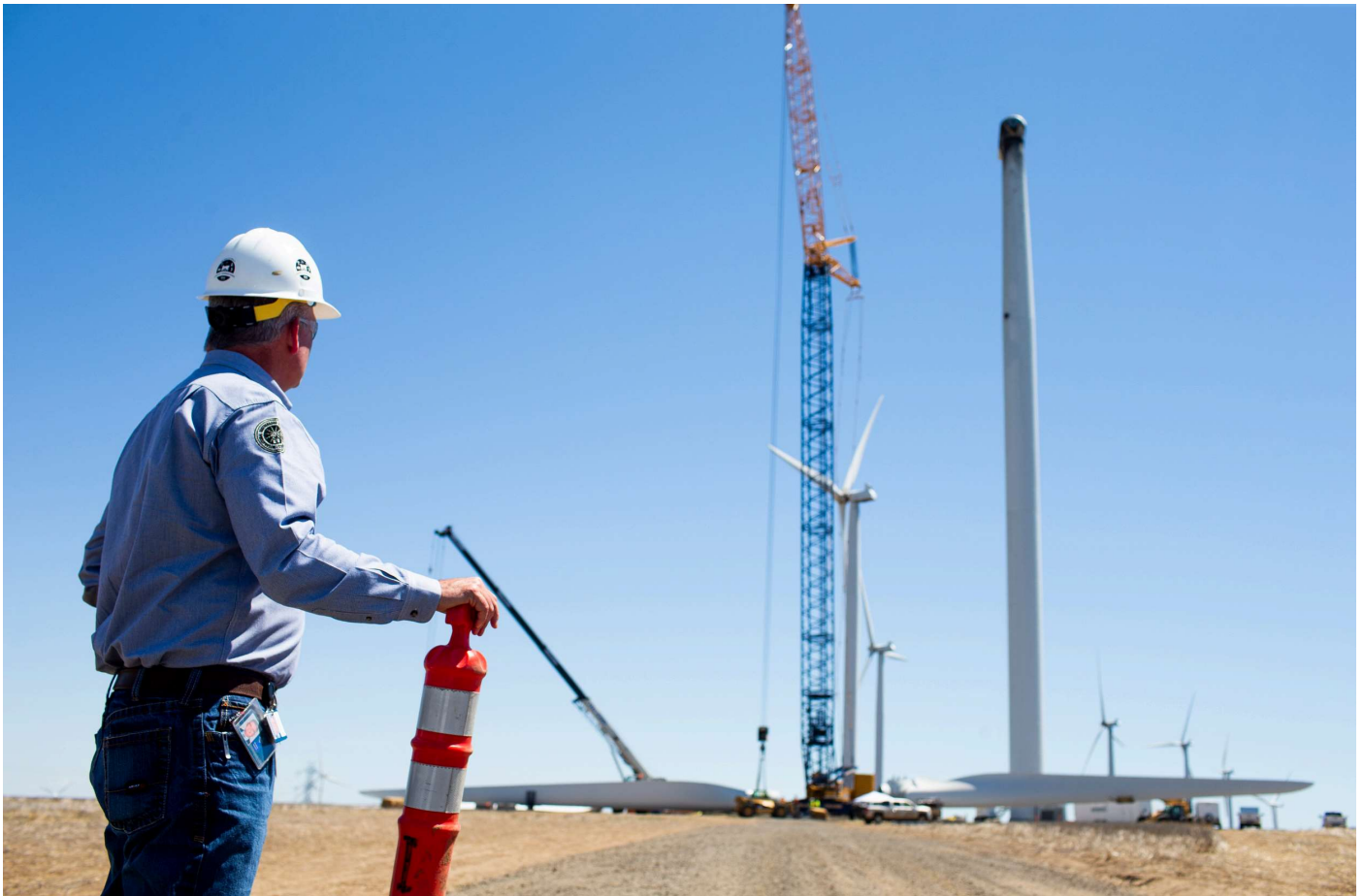
Brad Jenkins, PGE's vice president of utility operations, watches as workers install new blades in late June on the Vestas turbine that threw a blade on Feb 1.
