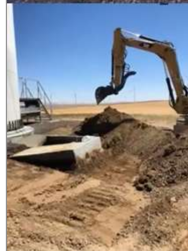
Screen shots of a ruptured transformer and the required cleanup of a transformer oil spill from a presentation that PGE made to state regulators in January about transformer problems at the wind farm.
