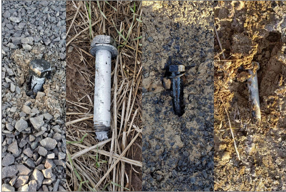
Broken blade bolts were scattered around turbine 71 at Portland General Electric's Biglow Canyon wind farm after the turbine threw a blade in the early hours of Feb. 1. Hours before the blade throw, a driver delivering fertilizer became stuck in close proximity to the turbine and had to be towed out. (Courtesy Kevin Massie)
