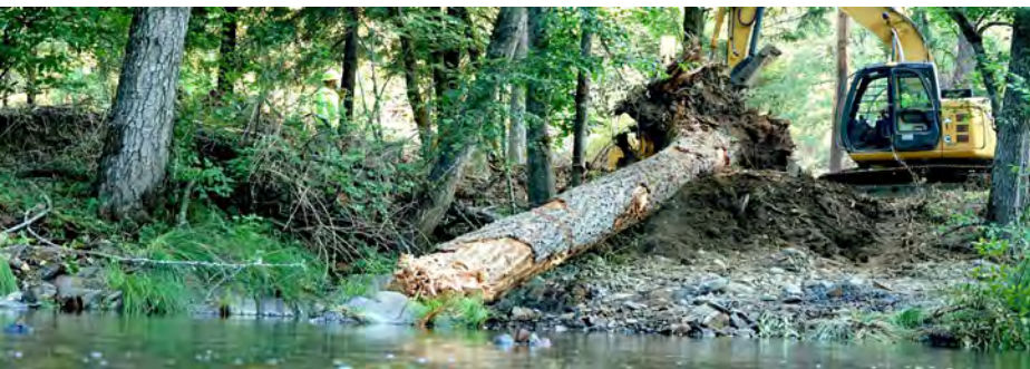
Lovelace dam removal and river restoration was the first BIL project in Oregon across the finish line
