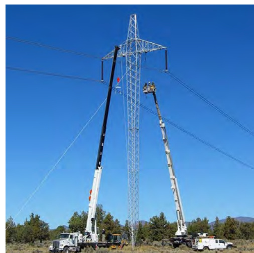
Crews from Central Electric Cooperative perform maintenance and repairs on high-voltage lines.
