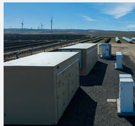
Portland General Electric’s Wheatridge Energy Facility includes battery storage.
