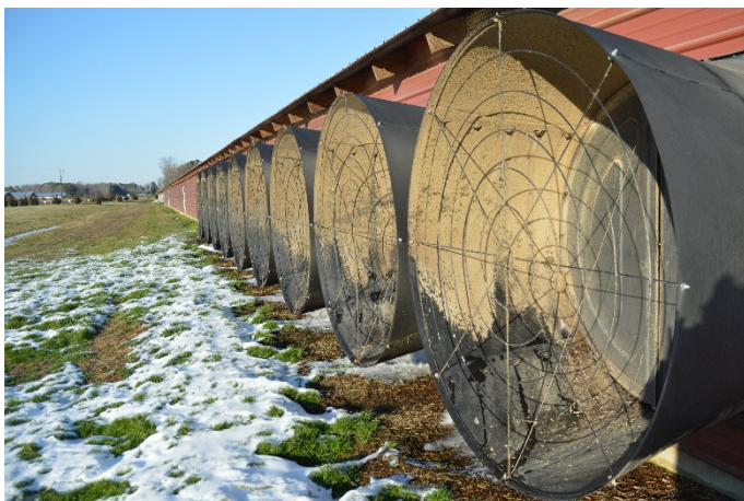
Exhaust fans on 600-foot-long chicken houses blow feathers, dust and particles of manure into Carlene Zach’s yard.
