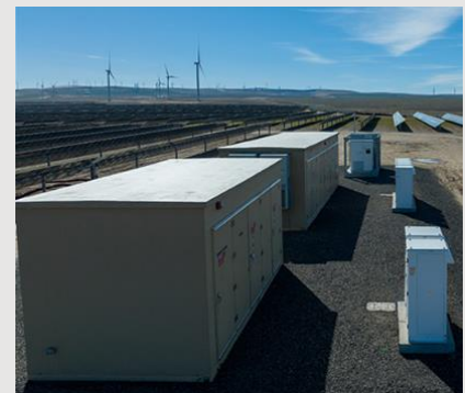
Wheatridge Facilities (PGE)
