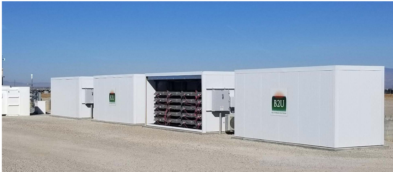
FIGURE 2: B2U STORAGE SOLUTIONS' STORAGE SYSTEM AT A SOLAR PV FIELD IN CALIFORNIA. THE CURRENT OPERATIONAL SYSTEM CAPACITY IS 8MWH AND WILL BE INCREASED TO 17MWH BY Q2 2022.
