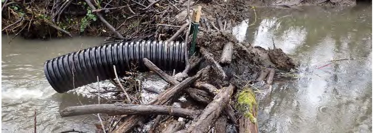
Outlet pipe of beaver pond leveler installed on Dunawi Creek to help reduce flooding of 53 rd Street.
