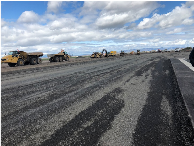
2017-2018 – Rehab Parallel Taxiway Design and Construction Total Project Cost: $2,996,664 ODA COAR Grant: $172,500
