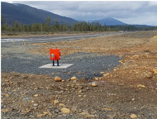
2017 – Airfield Lighting and Electrical Improvements (Design and Construction) Total Project Cost: $2,534,110 ODA COAR Grant: $140,212
