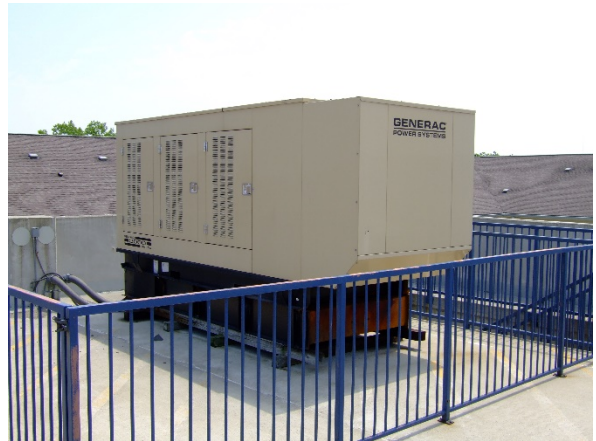
2020-Emergency Stand-by Generator at Emergency Operations Center Total Project Cost: $111,112 ODA COAR Grant: $100,000.00 (Not the actual generator, photo is an example)
