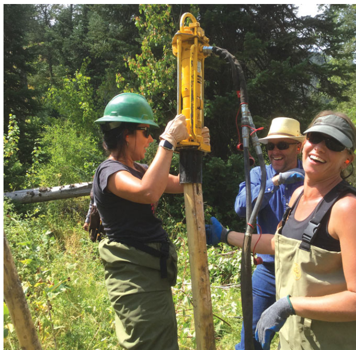
Staff from the USDA Natural Resources Conservation Service pound posts to build a beaver dam analog across Birch Creek in Idaho in 2016. The effort gave nine relocated beavers a head start to create their own dam complexes.
