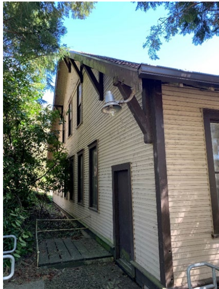
Clackamas Complex Building 4 Currently used by N Willamette District and Fish Research. Was the Hatch House for the former fish hatchery.
