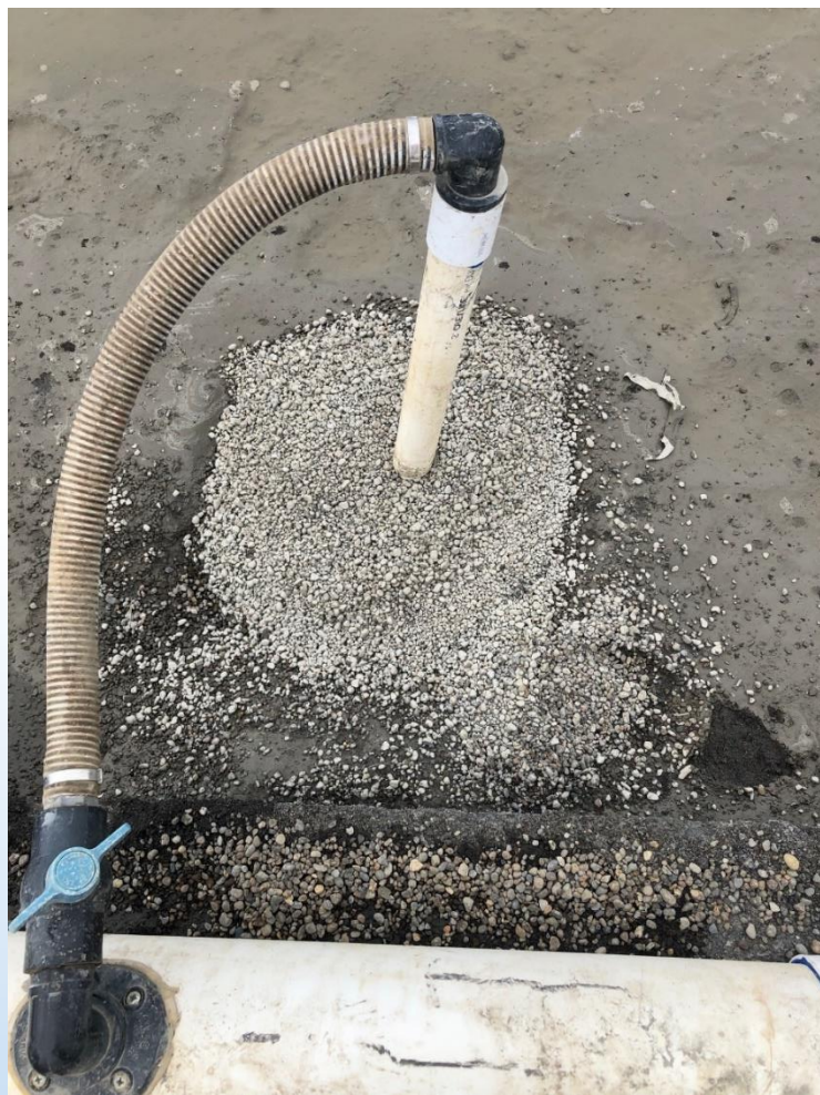
Improper seal: Wrong type of materials
