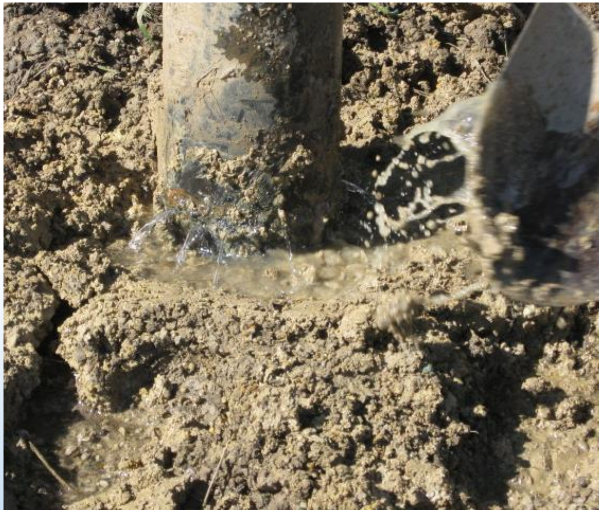
Bad weld allowing water to leak at joint
