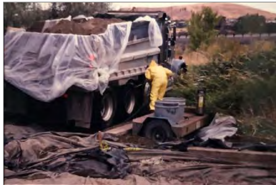
Workers in 1992 removed tons of soil contaminated by the rail tie plant at what is now the city's Riverfront Park.
