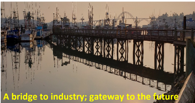
Holes in the existing pilings
