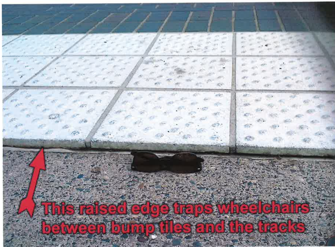
Figure 15. Bump tiles at Beaverton Transit Center showing a trap risk for wheelchair users
