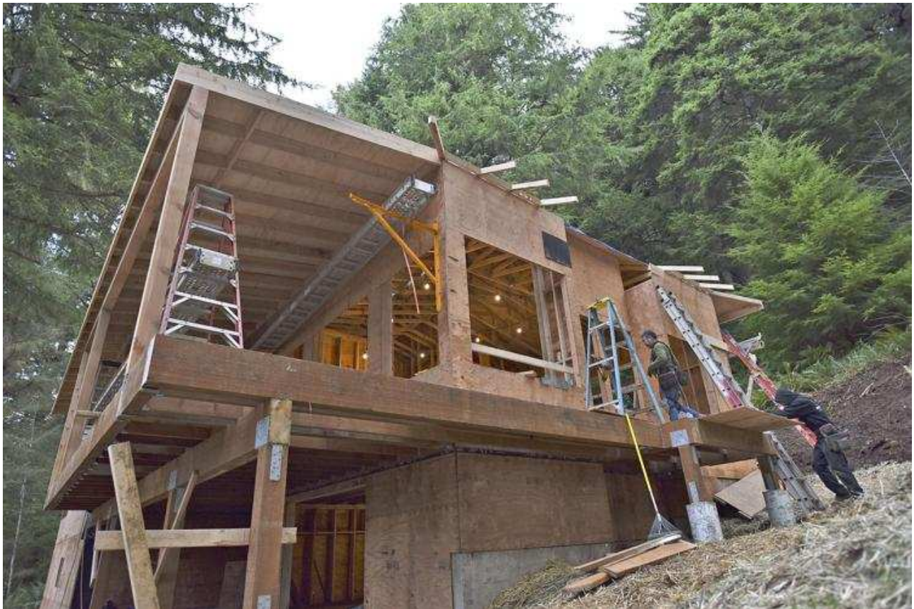
Construction workers build a home in the Falcon Cove area south of Cannon Beach.
