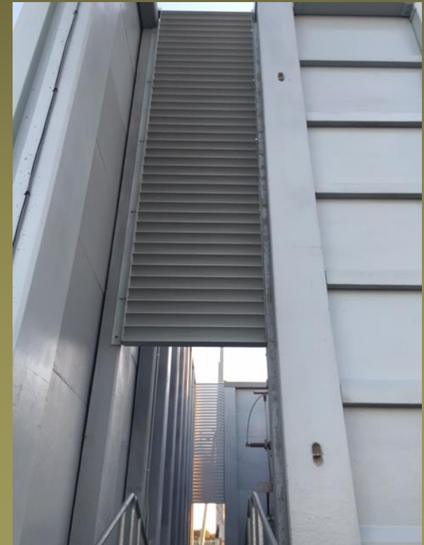
Transformer Protection Walls with Louver Line-of-Sight Protection
