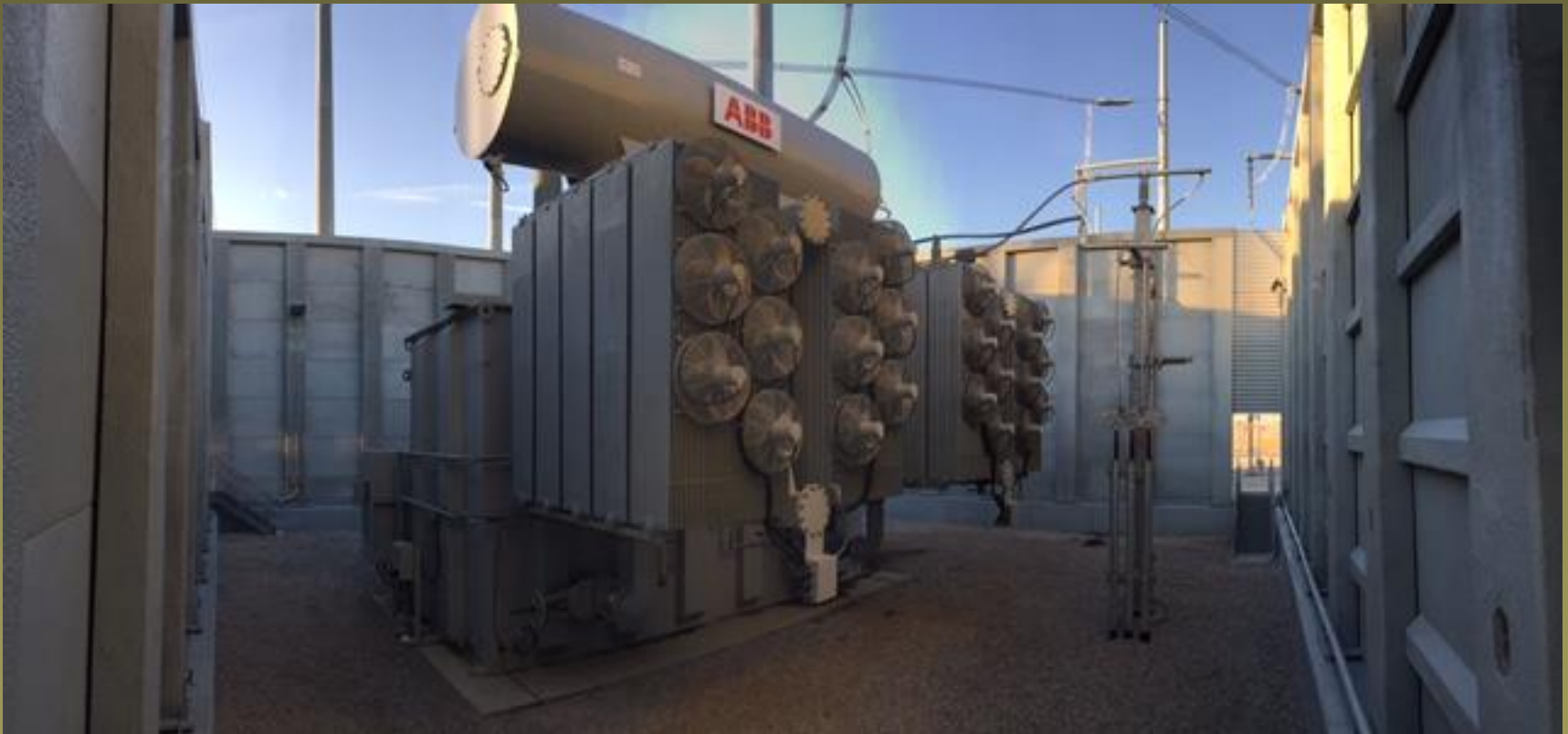
Transformer Protection Walls – Interior View
