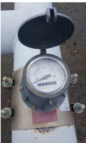
Broken water meter
